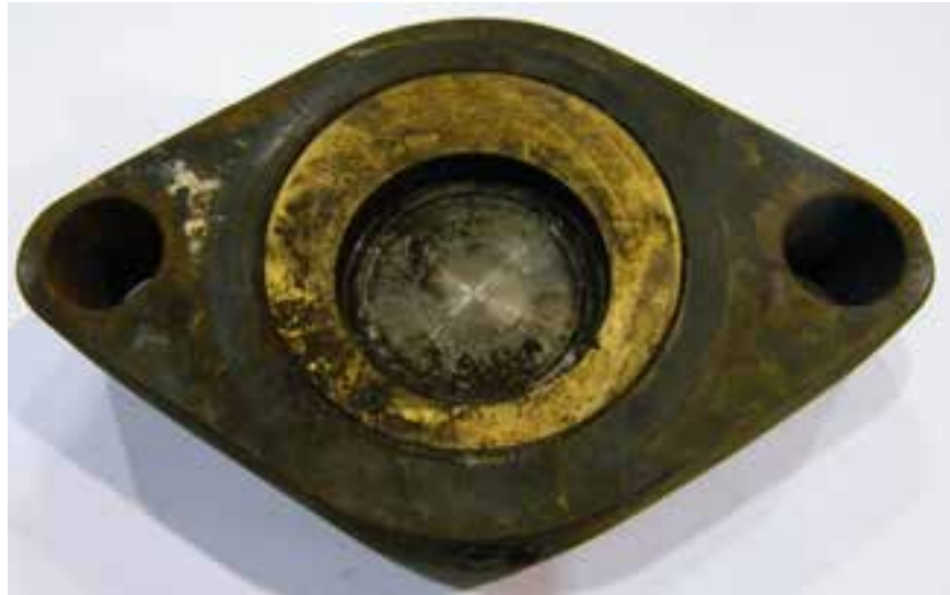
(a) Viewing from the inlet side of the check valve
