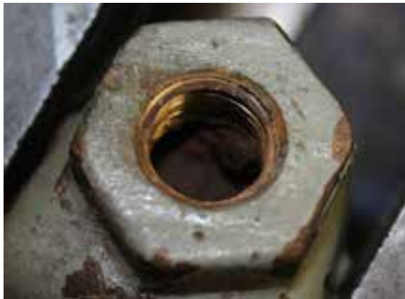
(a) Inside view of the valve from the exit hole after removal of the outlet pipe
