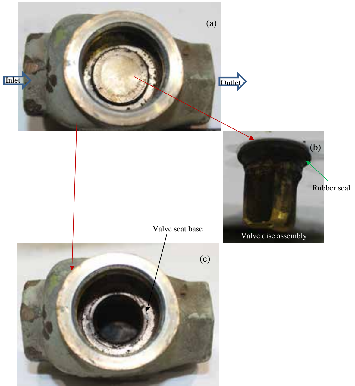
Figure 13: Photos of the inside structure of the dead engine pressure regulating valve from locomotive unit CEFX-3166
