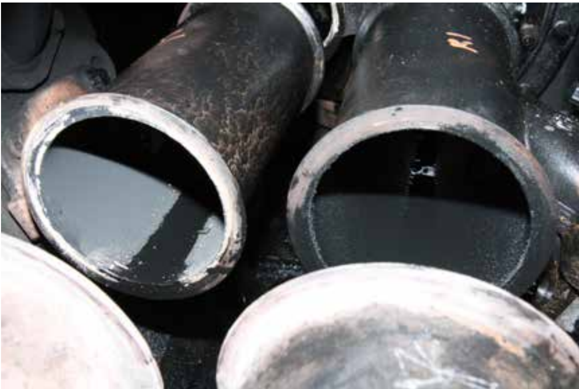
Figure 10: Exhaust manifold bodies for cylinders L1 and R1 showing oil buildup
