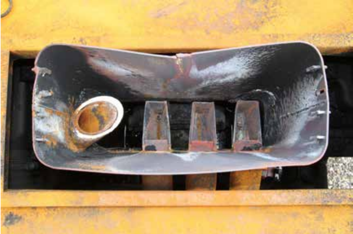
Figure 3: View inside the exhaust stack showing surface of oil/water mixture Aspirator venturis are visible
