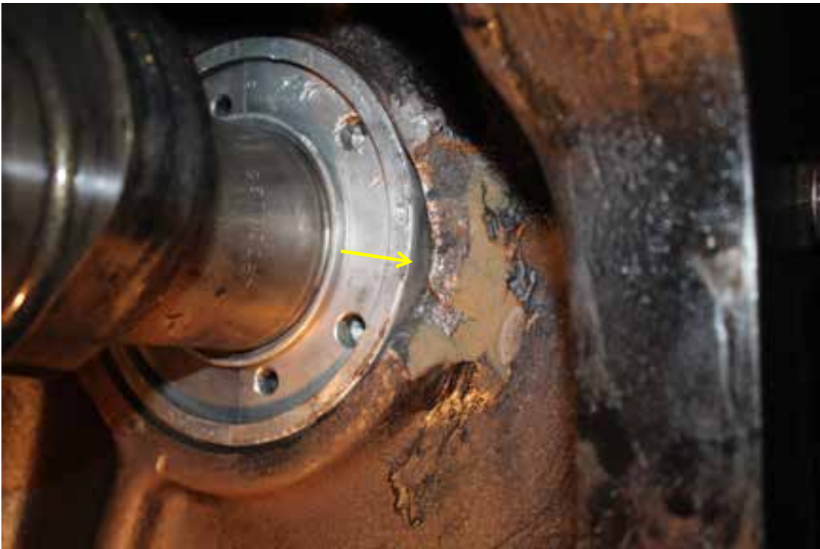
Figure 39: Substitute bearing in R4/R5 position showing unsupported bearing area (arrowed)
