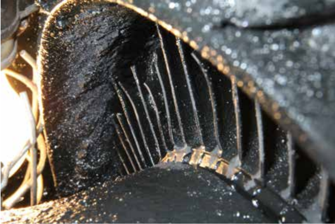
Figure 7: Bent and broken turbine blades in the turbocharger
