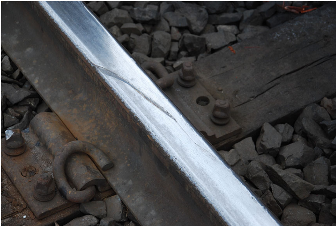
Figure 3. Flange mark left by the train on the rail (Mile 0.40, Red Deer Subdivision)
