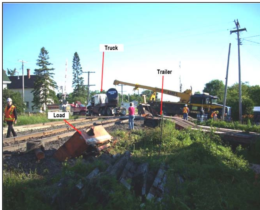
Photo 4. Damage to lowboy truck and load
