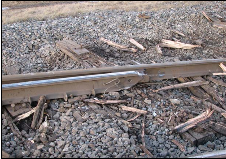
Photo 1. Track ties beneath the heel block joint
