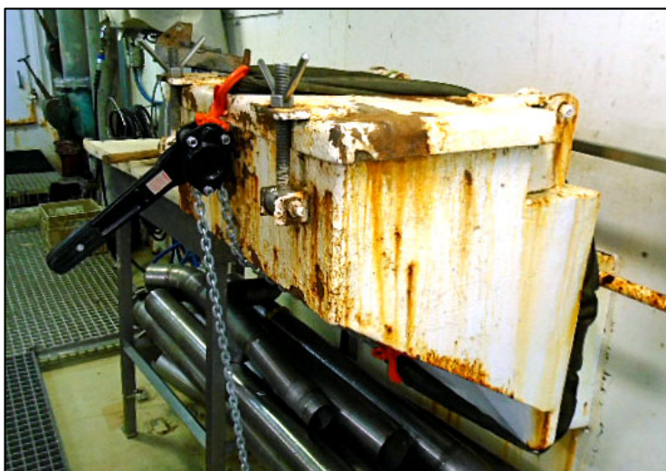
Figure 4. Chain hoist used to secure hatch (Source: Nataaaqnaq Fisheries)
