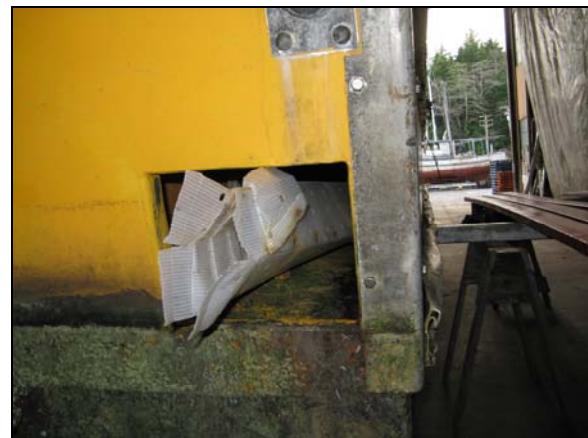
Photo 4. Starboard freeing port with protruding cone
